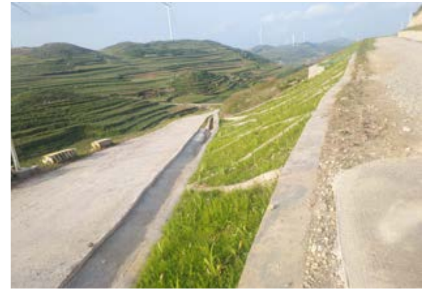
Longyuan Guizhou Company Weining Xiaohai Wind Power Project implemented the principle tht water and soil conservation construction designs, constructs and puts into operation with the major engineering construction. The picture shows the water and soil conservation governance achievement demonstration.
